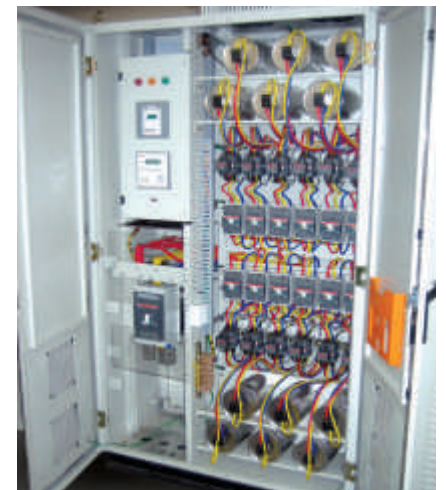
LVAS-C System (with MPP) capacitors
